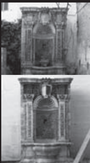
Before and after - One of the fountains, nearing its completion stage. The treatment involved the intervention of plastic repair, pointing and lime washing
