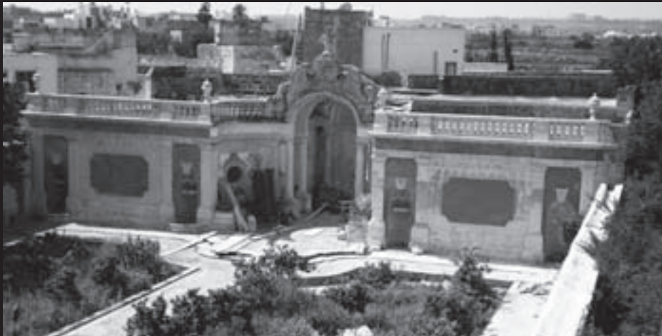
Elevation of nymphaeum prior to initialisation of the restoration and conservation project
