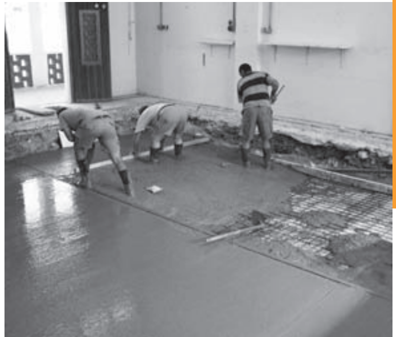
Above : Reinforced steel concrete foundation to support the loads exerted by the dynamometer and scissor lift.
