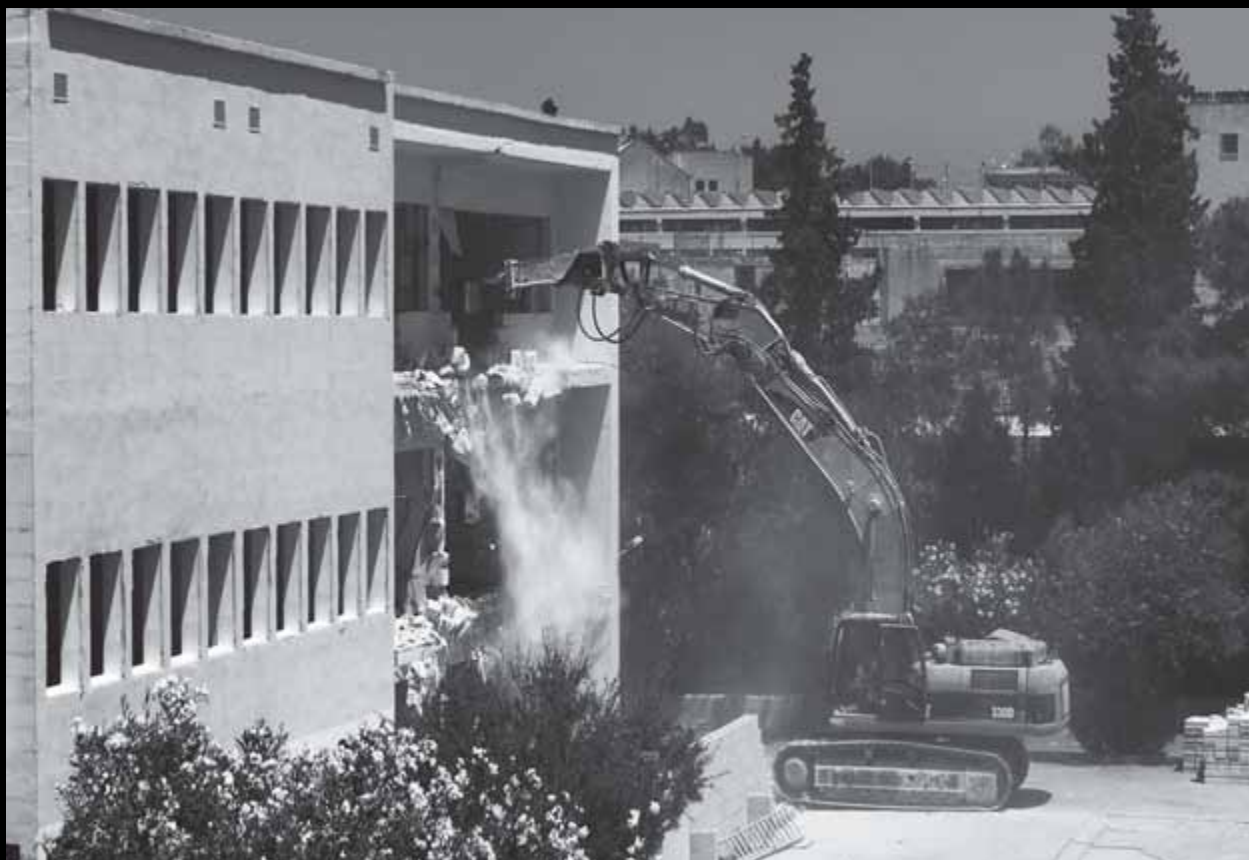
Pulling down Block B (IBAC) to make way for the new Institute of Applied Science
